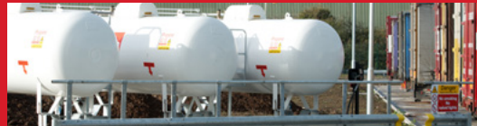
UTILITIES & CRITICAL INFRASTRUCTURE
